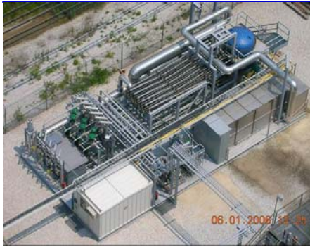
ITM Air Separation 5 TPD test at APCI's Sparrows Point gas plant
